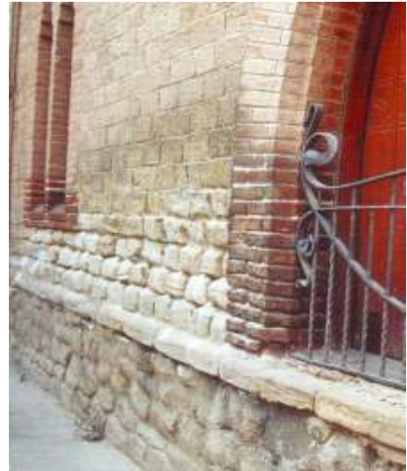
Rising Damp in stone wall ▶
