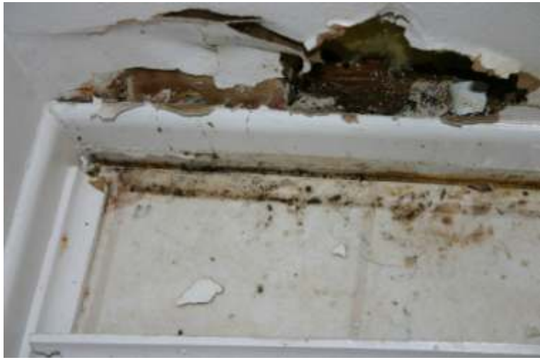
Rotting skirting boards and peeling paint due to rising damp ▲
